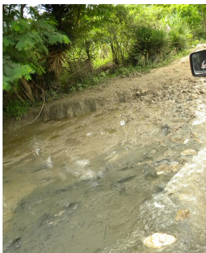
The road to Bois l'Etat at a point of inundation
